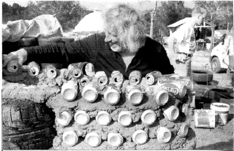
Michael Reynolds and friends at work. Note used tires—the basic building-block, front-left and background—filled with dirt compacted with a long-handled mallet.
